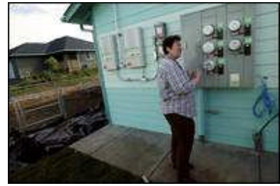
Jody Ahlstedt, a program director for Umpqua Community Action Network, shows off the solar energy converters next to the meters at Mariposa Villa in Winston. Behind her is the unfinished toddlers play area.
